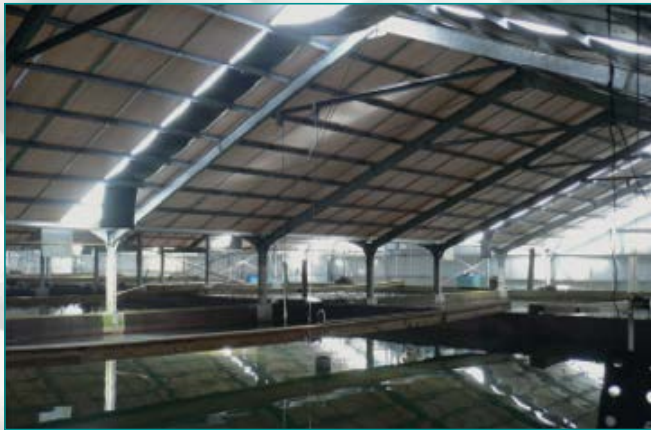
Fish farm facility
